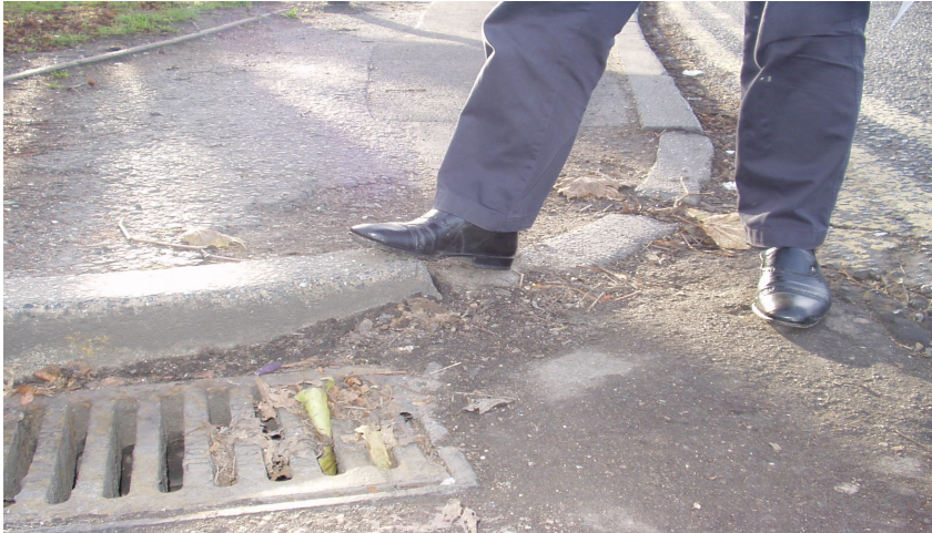
Broken and uneven surfaces can be dangerous for the elderly and vulnerable residents
